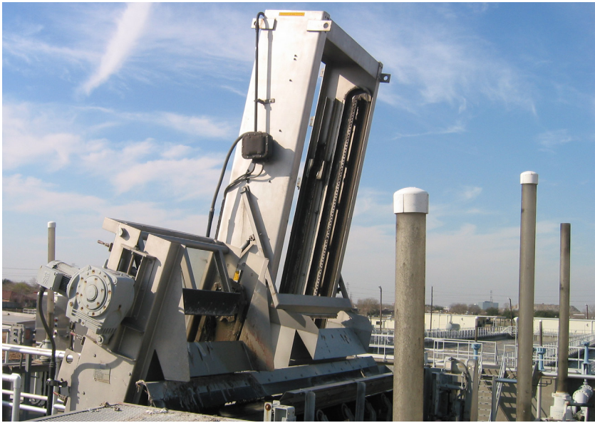
The Mahr Bar Screen operated for 10 years of run time with no chain, sprockets, or lower bearings requiring replacement.
