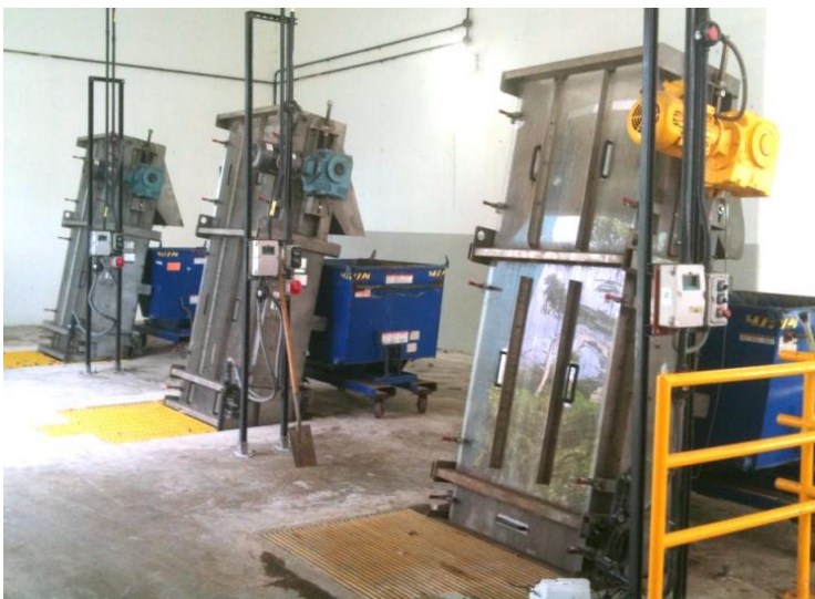
Three Mahr Bar screens installed at Caguas WWTP in Puerto Rico.
