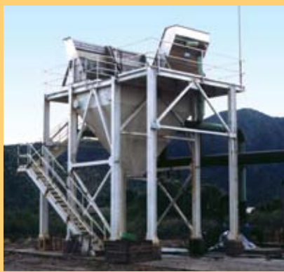
Three TS 2000s handling water runoff at a paper mill.
